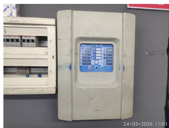
Alarm control panel.jpg
