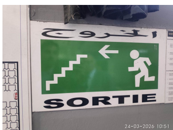
Signing of emergency stairs.jpg
