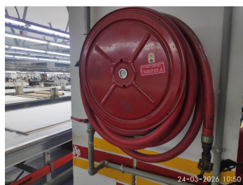
Fire hose pipe_1.jpg
